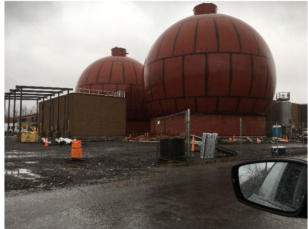
Figure 1: Aerial View of Oneida County Sewer District WPCP (left) and Digester Construction Progress (right)
