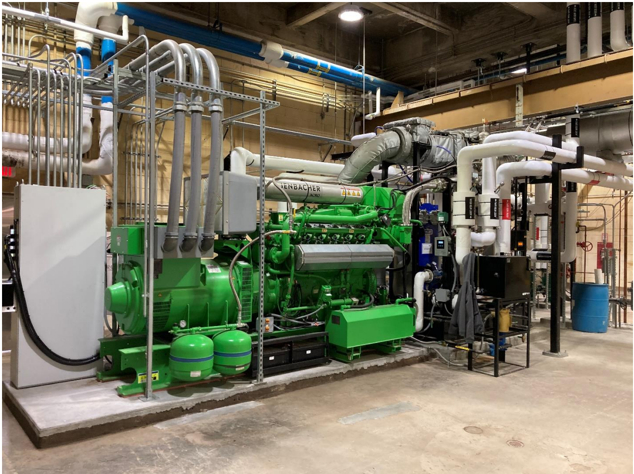
Figure 7 Biogas Engine Generator with Heat Recovery
