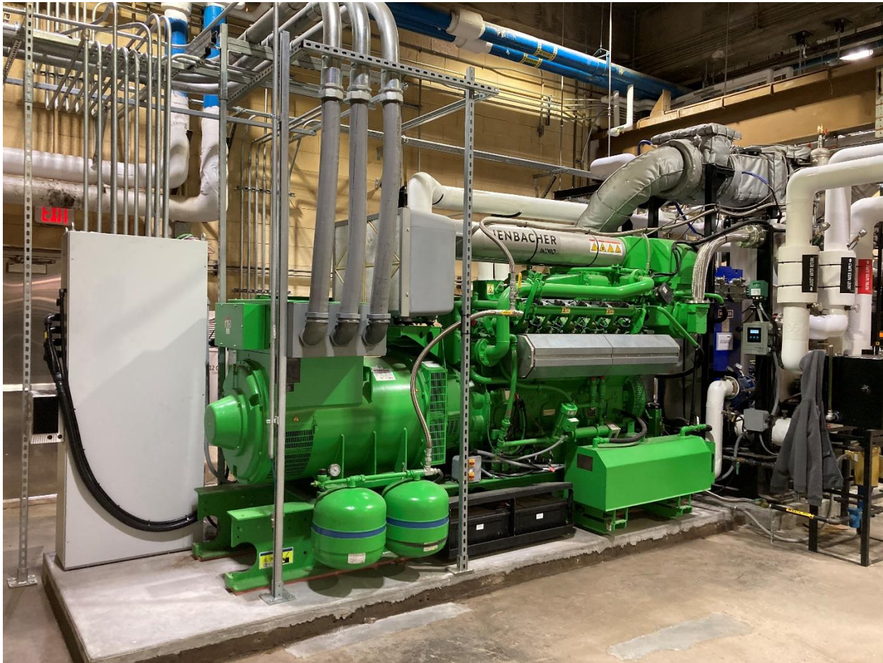
Figure 1: GE 633 KW Engine/Generator
