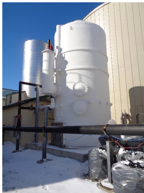
Figure 3: Biological scrubber system
